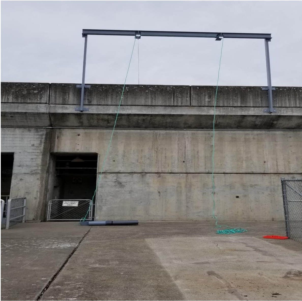
Hoist frame at east fishway exit for tribal lamprey trapping to lift to forebay deck
